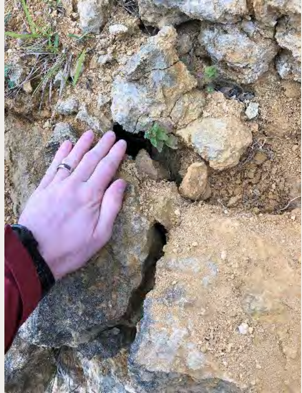
Photograph 58: Photograph of open voids and open joints overprinted by spalling. Spalling controlled by frost weathering. Photo looking 130°.
