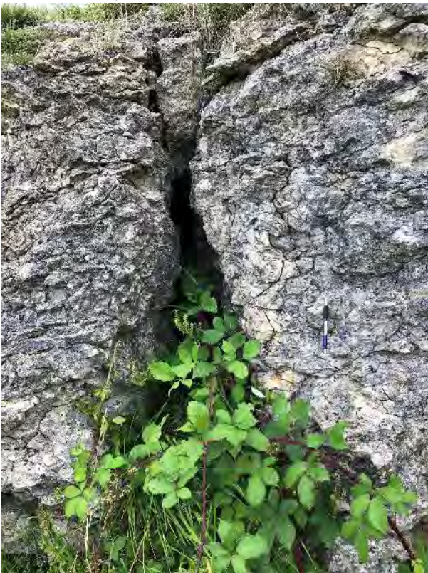
Photograph 13: IMG_3259. Photograph of small (circa 100-300mm wide) gull fissure within limestone (IO) exposure on escarpment slope. Photo looking 020°.
