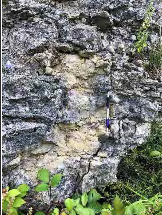
Photograph 12: IMG_3255. Photograph of fresh rockfall scar from limestone (IO) exposure. Photo looking 100°.
