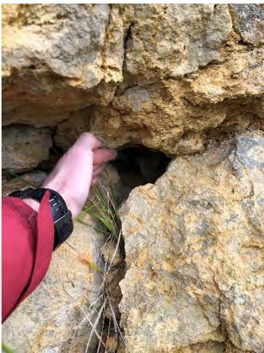
Photograph 59: Photograph of open voids and open joints overprinted by spalling. Spalling controlled by frost weathering. Photo looking 130°.
