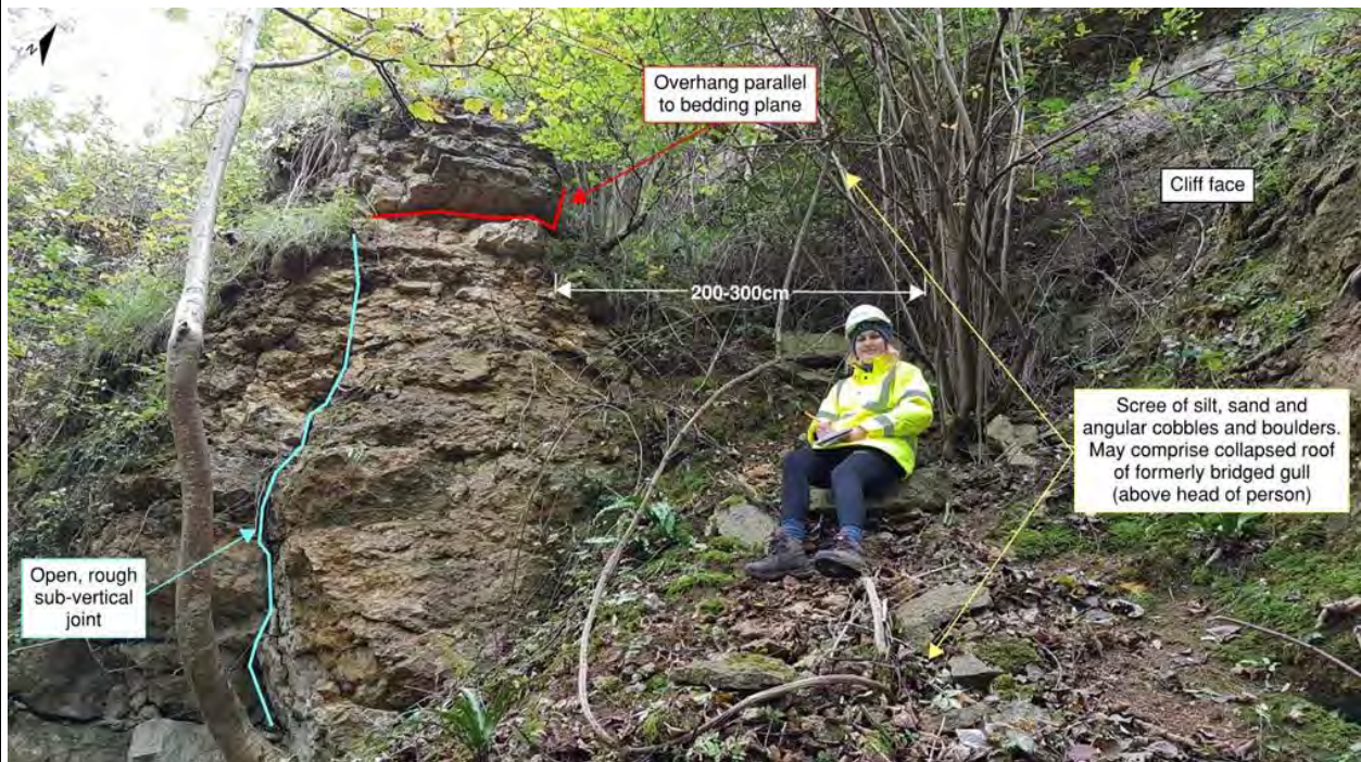
Photograph 62: Photograph of active material gully formed in collapsed joint (width 2-3m). Photo looking 340°
